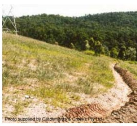
Earth-lined catch drain
